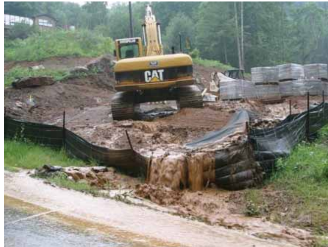
Figure 9-3 Example of an Erosion and Sediment Control Failure.
