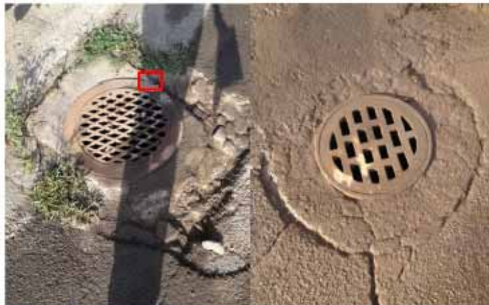
Figure 2—Two of the outdated and inefficient catch basins on Prospect Hill Ave.
