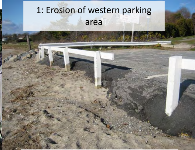
2. Erosion from parking lot runoff
