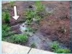
Problem Deep gullies are forming within a rain garden.
